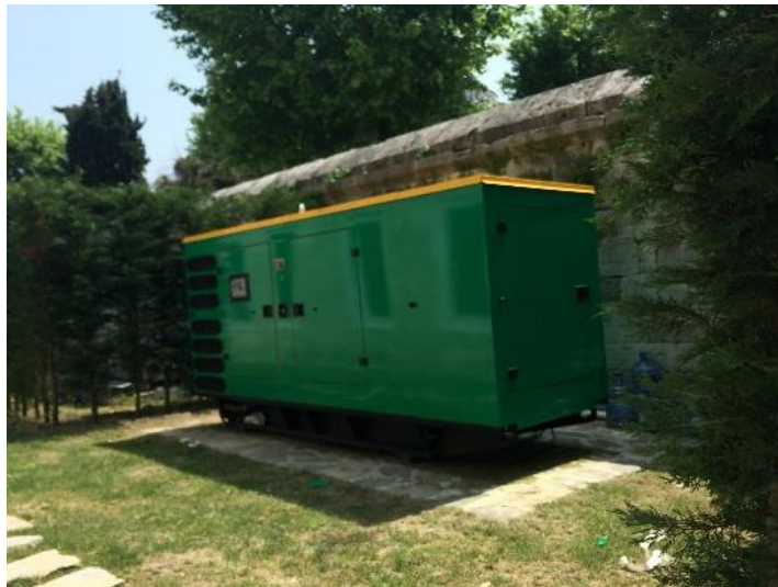
Figure 3.319. Generator at the back garden, 2015
