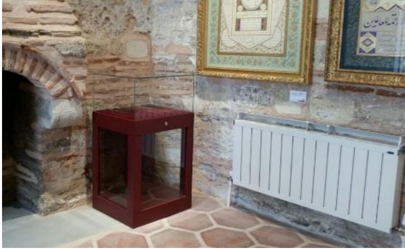
Figure 3.247. Radiator in a room in Siyavuş Paşa Medrese, 2016
