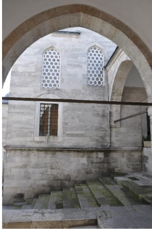
Figure 3.184. Improper installations after restoration on the façade of the classroom, 2016
