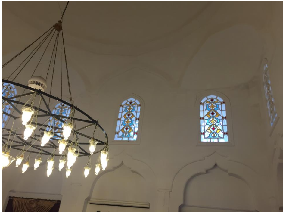
Figure 4.20. Ornamented architectural elements in the transition zone of the classroom of Rüstem Paşa Medrese in 2015
