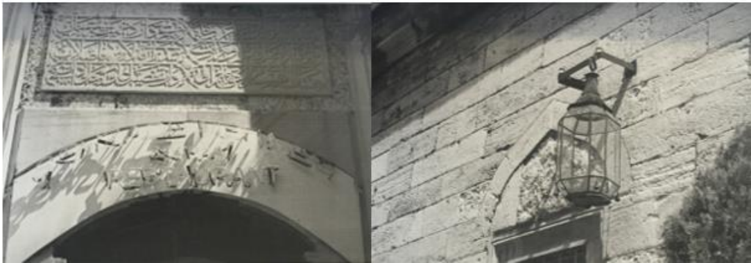
Figure 3.100. Interventions nailed to original masonry of Şehzade Medrese in 1990's (archive of DGF)
