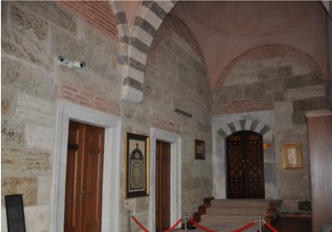
Figure 3.315. Electric installations on revak walls, 2015
